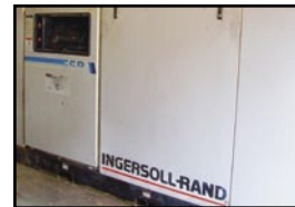
100 HP Ingersoll-Rand Air Compressor
